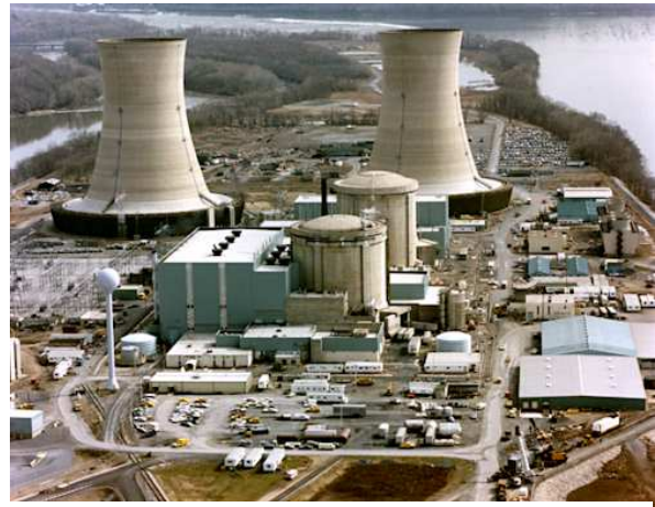
The Three Mile Island nuclear generating station before the 1979 accident
